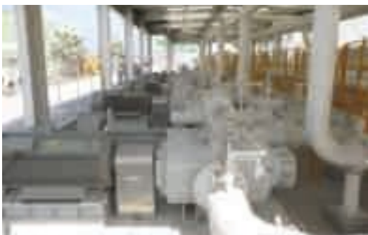
Numerous Twinro pumps installed at a fuel oil terminal in the UAE
