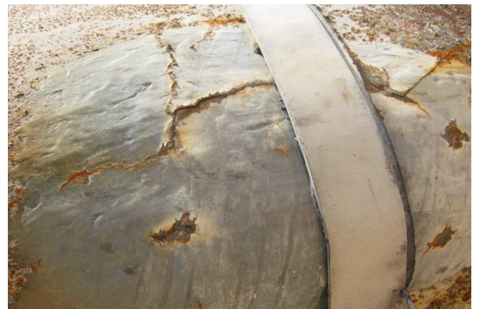
Stress corrosion cracking visible on trouserleg
