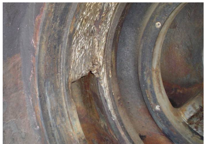
Erosion at cutwater
