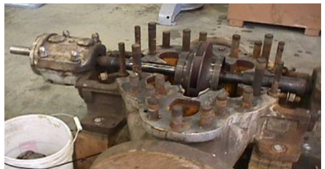
Top half of casing removed to see condition of the rotor.
